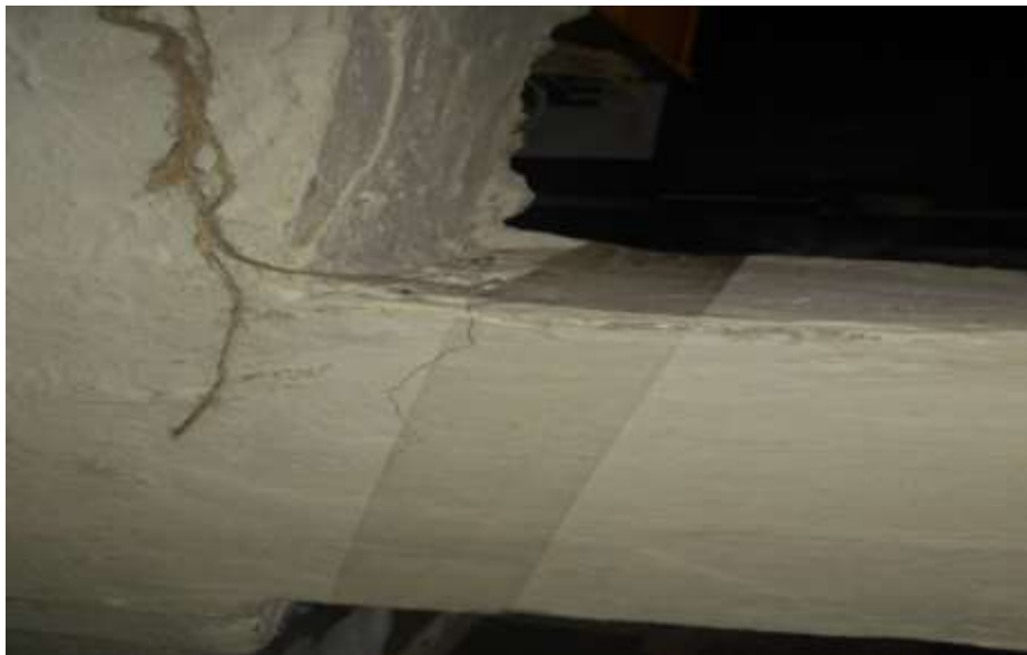
Figure 5: Shear crack at the joint in BC 3
