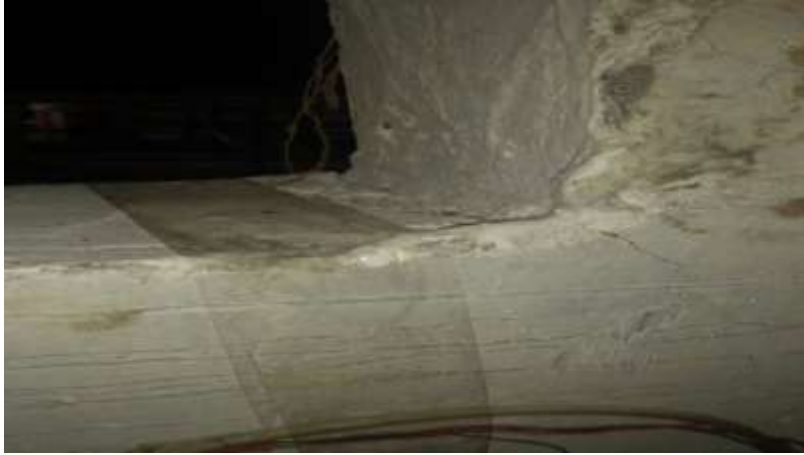
Figure 6: Shear crack at the joint in BC 4
