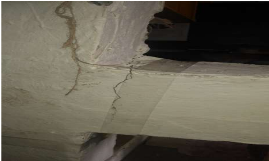
Figure 4 Shear crack at the joint in BC 2
