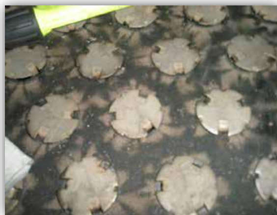
Figure 10: Undismantled tray after online cleaning [7]
