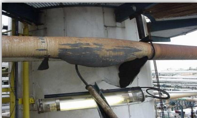
Figure 8: Rupture in butadiene reboiler in Lavera Petrochemical Complex in December 2000 [4]
