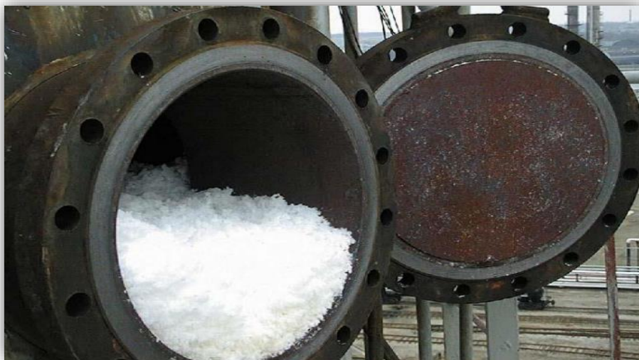
Figure 5: Popcorn polymers in a manhole of butadiene extraction unit [6]
