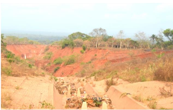
Figure 3: Photo of Jatuu Road Gully Site in Edo North
