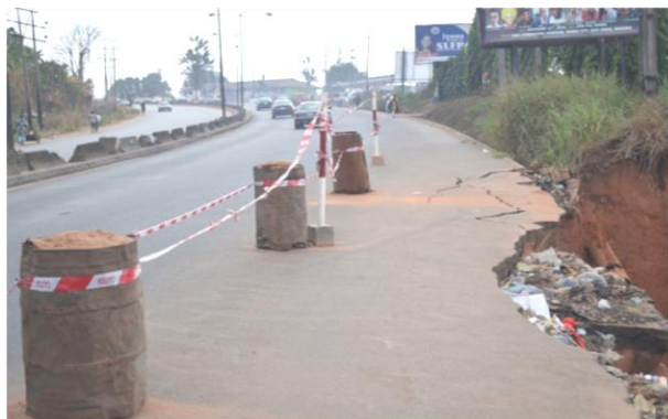
Figure 4: Photo of Ikpoba Slope Gully in Edo South Threatening the Highway
