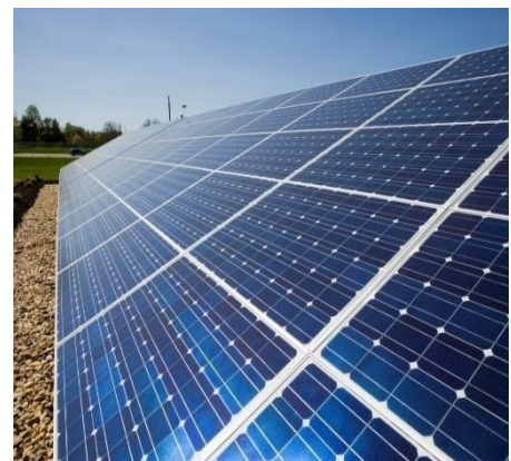
Figure1: Solar PV panel
